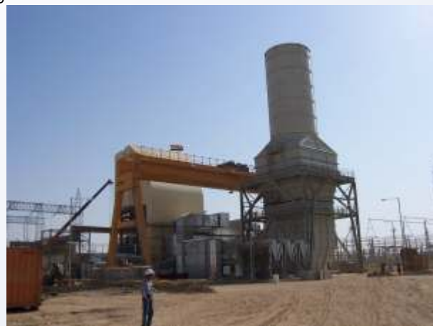
A 130/25/15 ton, 105 foot span, double girder gantry crane installs and services turbines at an overseas power plant. The crane uses three EMH engineered hoists.
