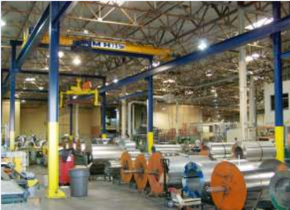
A 7.5 ton NOMAD system at a Western manufacturer of ducting.
