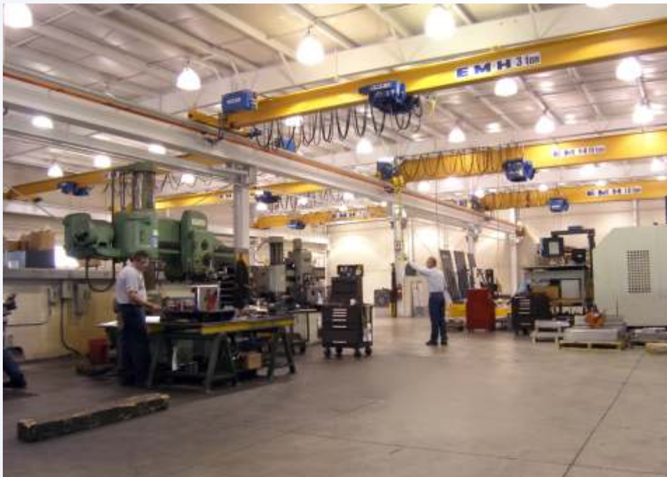
Multiple standard single girder cranes with capacities from 3 to 10 tons provide convenient access to lifting at a Midwestern machine shop.
