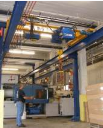
A NOMAD System at a Midwestern manufacturer of industrial containers was installed on a 182 foot freestanding runway located between concrete building supports.
