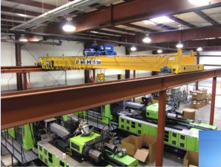
A 15 ton double girder free standing system at a plastic injection mold plant in Northeastern Ohio.
