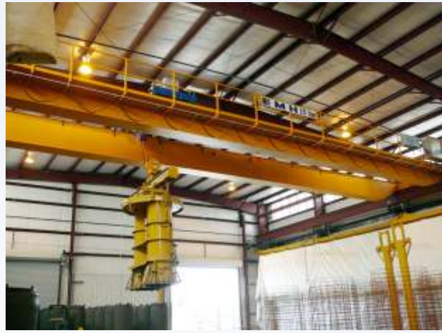
EMH is experienced in building cranes for the concrete industry. The crane above is in a high production concrete pipe facility.
