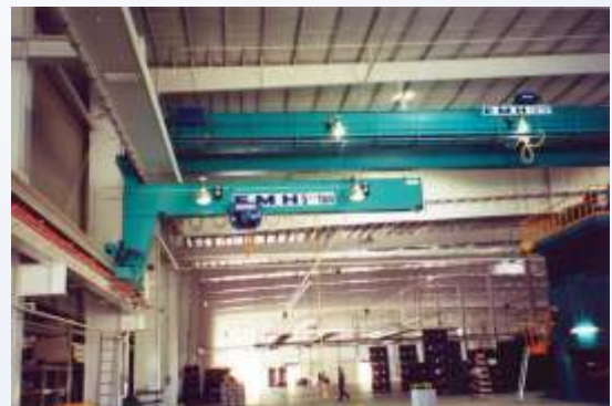
Above: Wall traveling jib crane.
