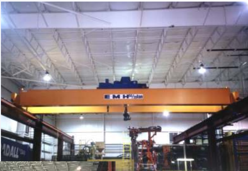
This double box girder crane features a 50 ton main hook and 20 ton auxiliary hook to lift and maneuver large molds at a Midwest automotive plastics facility. The crane is supported by a 350 foot runway, completely designed, manufactured and installed by EMH. The crane and runway are completely free standing because the original building structure could not support an overhead crane.
