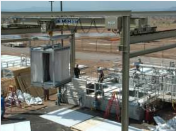
A NOMAD Free Standing Crane system is used outdoors at this Western water treatment plant. The crane lifts and changes filters.
