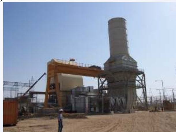
A 130/25/15 ton, 105 foot span, double girder gantry crane installs and services turbines at an overseas power plant. The crane uses three EMH engineered hoists.
